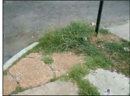
Broken, overgrown sidewalks are not ADA compliant
