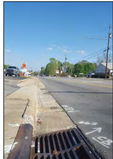
Improperly installed drainage grates are extremely hazardous for bicyclists.
